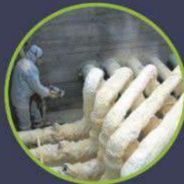
Corrosion detection in pipes and pipelines in PPU insulation
