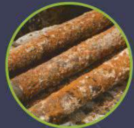
Corrosion areas detection in pipes through rust without stripping
