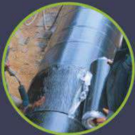
Corrosion detection in 3-Layer Polypropylene Coated pipes and pipelines
